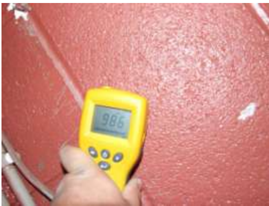
Protimeter reading 98% on interior wall
